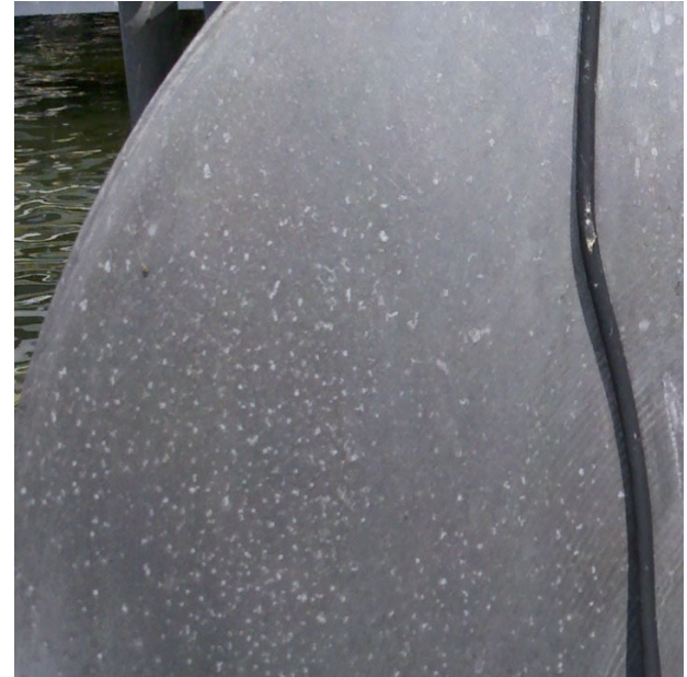
This boat hull is in the early stages of corrosion and corrective action should be taken to prevent any further damage. Photo by Jim Donahoe, used with permission.
